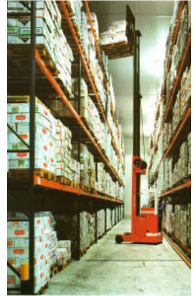
Even a warehouse this large can be made fireproof.
